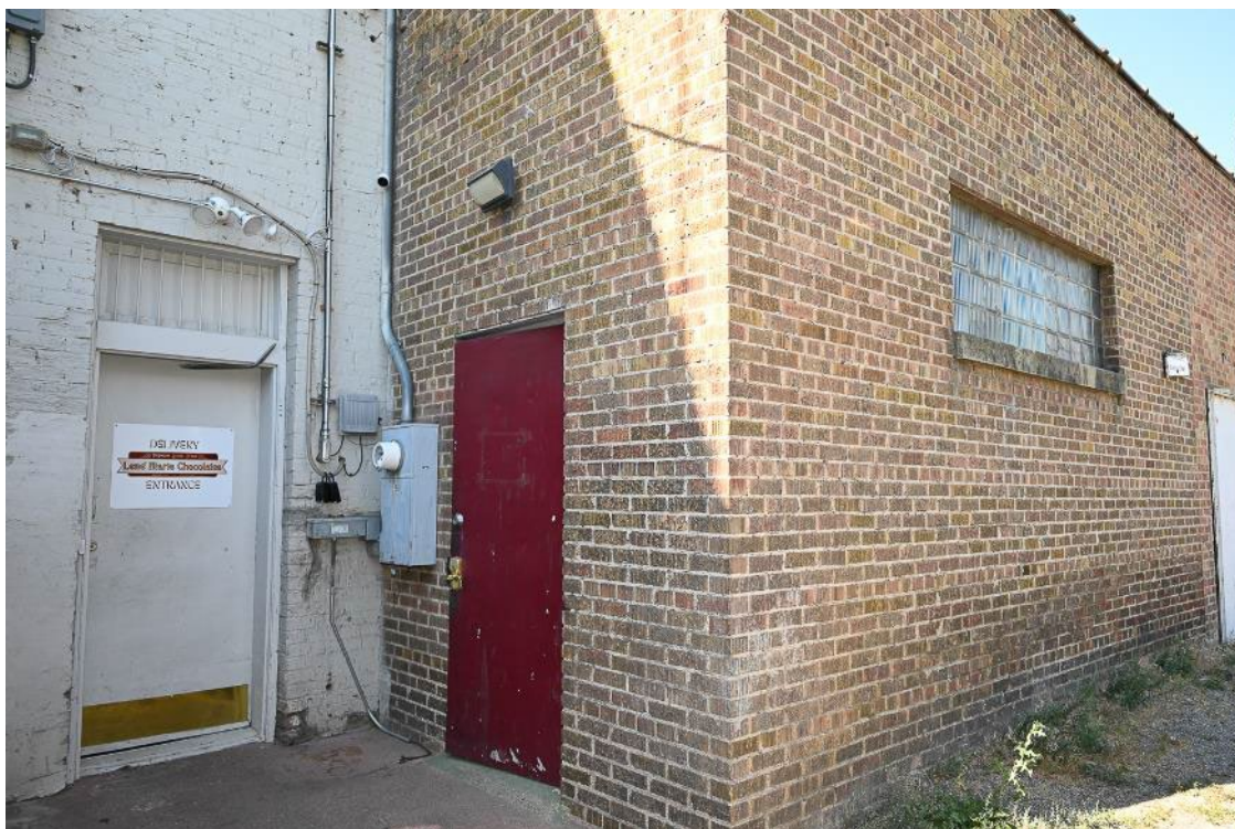
Photograph 8: North and east elevations of addition and rear entry. Camera facing southwest.
