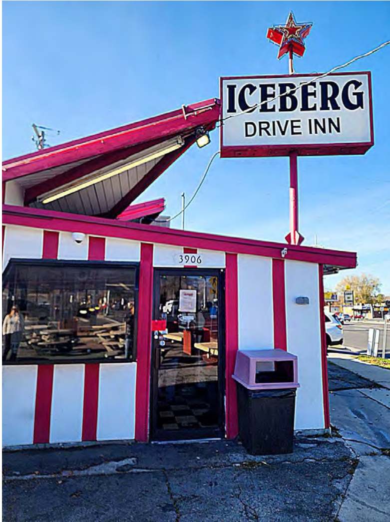
Photograph 7. Exterior, east (main) façade detail of eaves and sign. Camera facing northwest.
