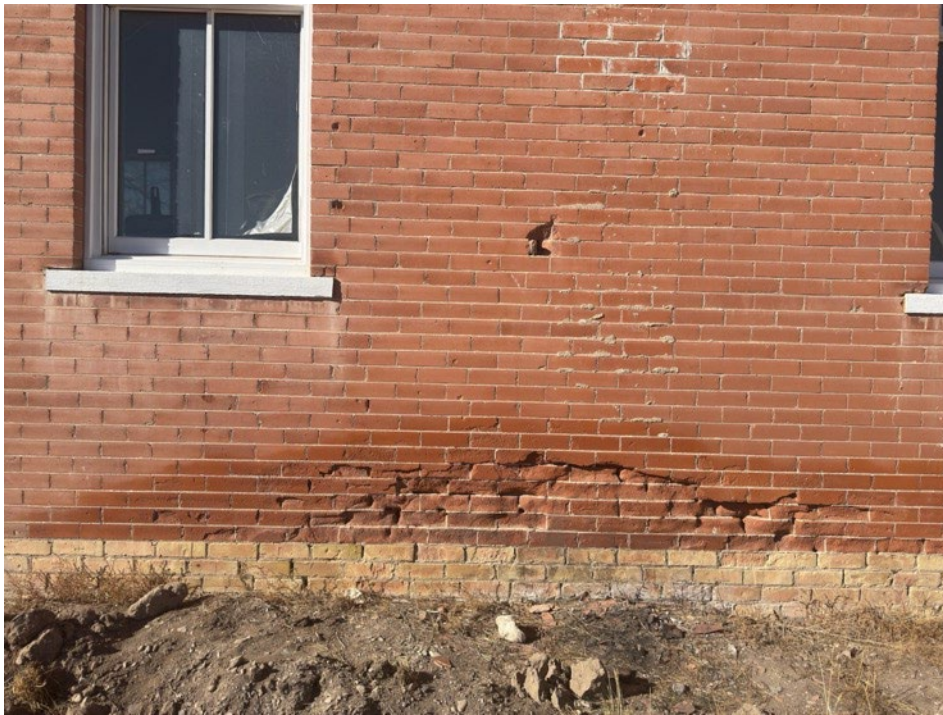
Photograph 12 of 19. Exterior, detail of brick deterioration, east facade. Camera facing west.
