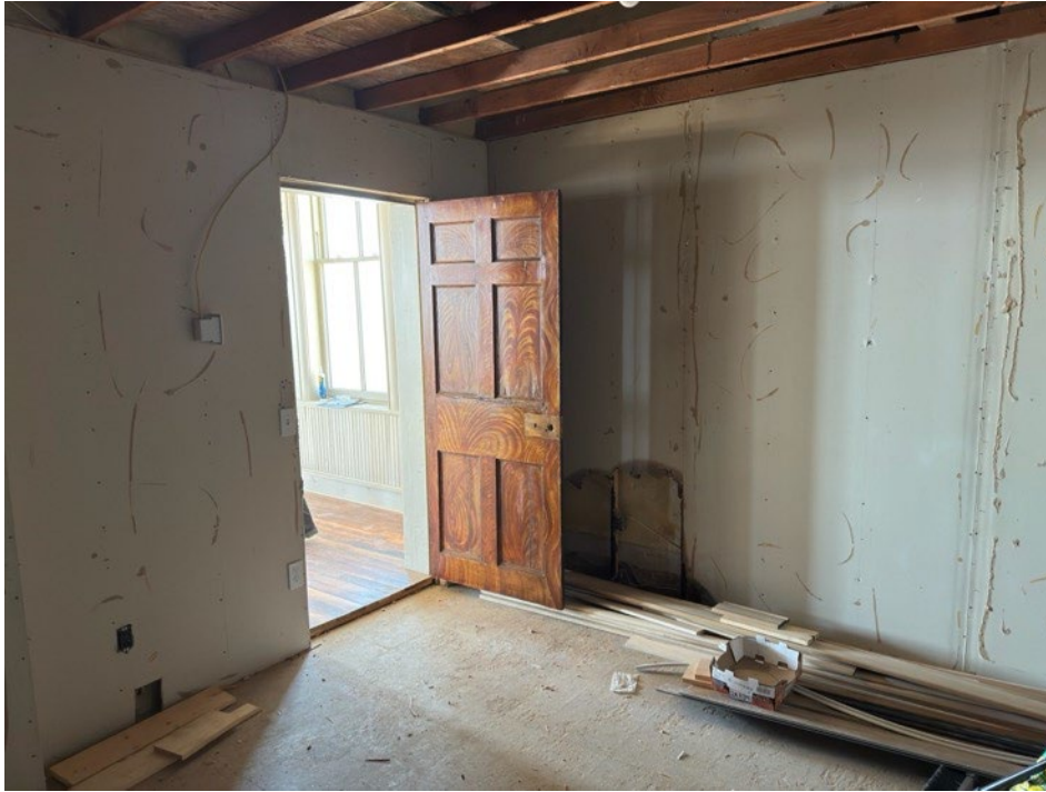
Photograph 17 of 19. Interior, vestry addition, detail of removed panels, and exposed rafters. Camera facing southwest.
