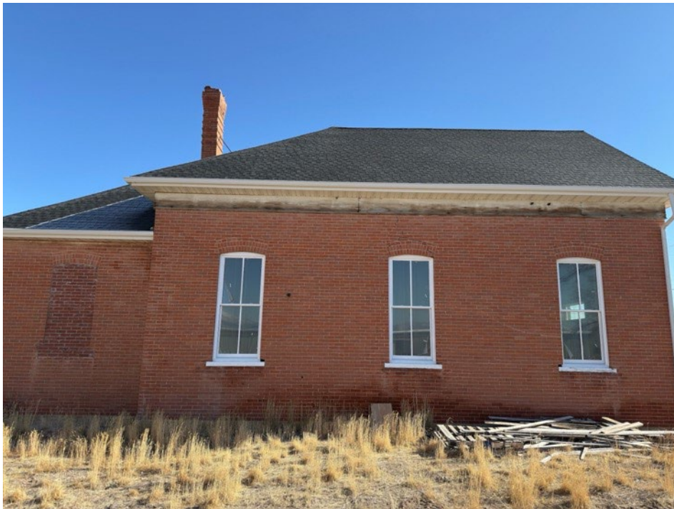
Photograph 6 of 19. Exterior, west facade. (Property boundary created a limitation to a clearer straight-view of this façade.) Camera facing east.
