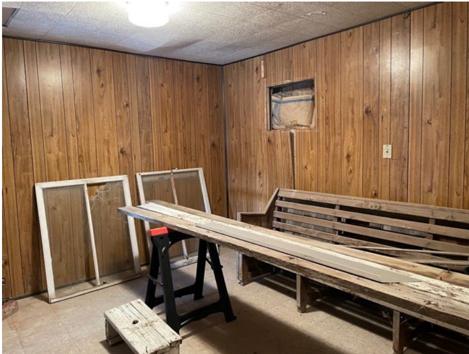
Figure 14 of 14. Interior of vestry prior to renovations, ca. 2022. Note the wood paneling installed by Beehive Telephone Company in the 1980s. Camera facing northwest. Source: Clover Church Restoration Committee.
