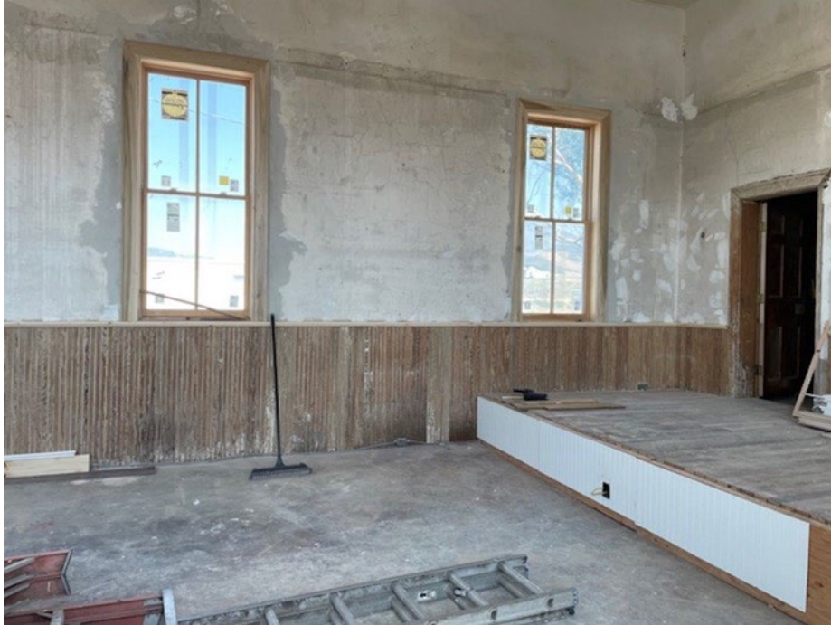
Figure 13 of 14. Interior renovations to the west façade and stage reconstruction, ca. 2022. Note the replacement windows and new stage. Camera facing west. Source: Clover Church Restoration Committee.
