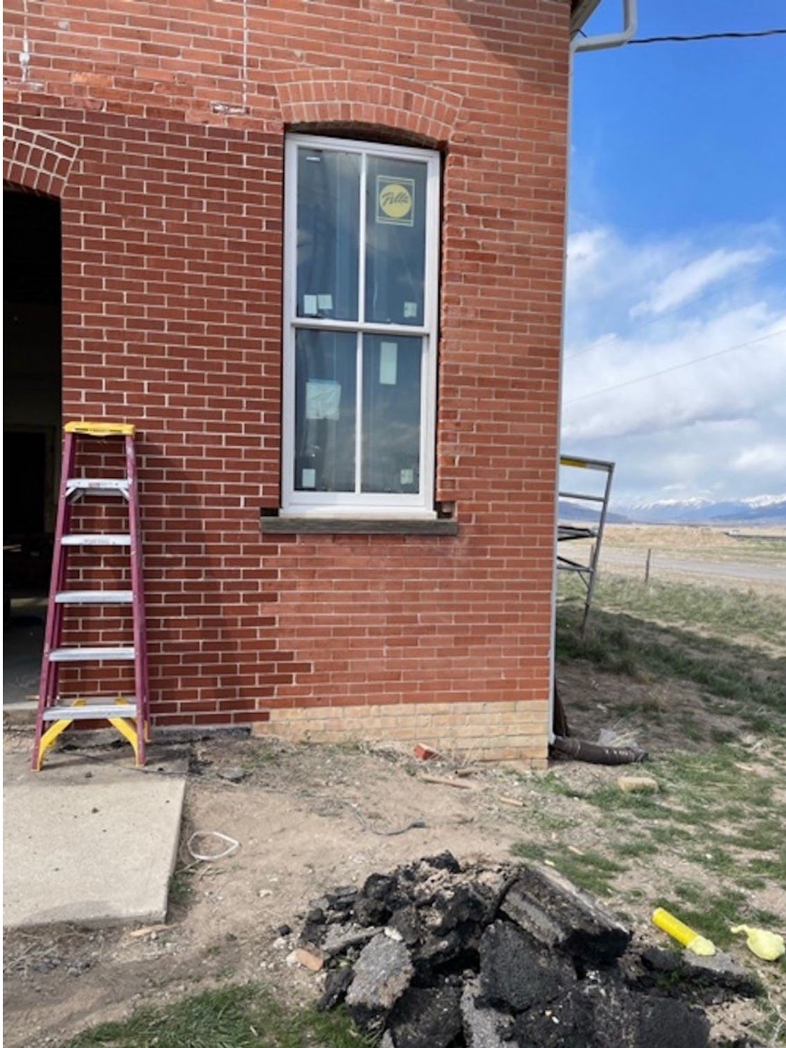
Figure 10 of 14. Restored brick and masonry on the Clover Meetinghouse main (south) façade, ca. 2022. Camera facing north. Source: Clover Church Restoration Committee.
