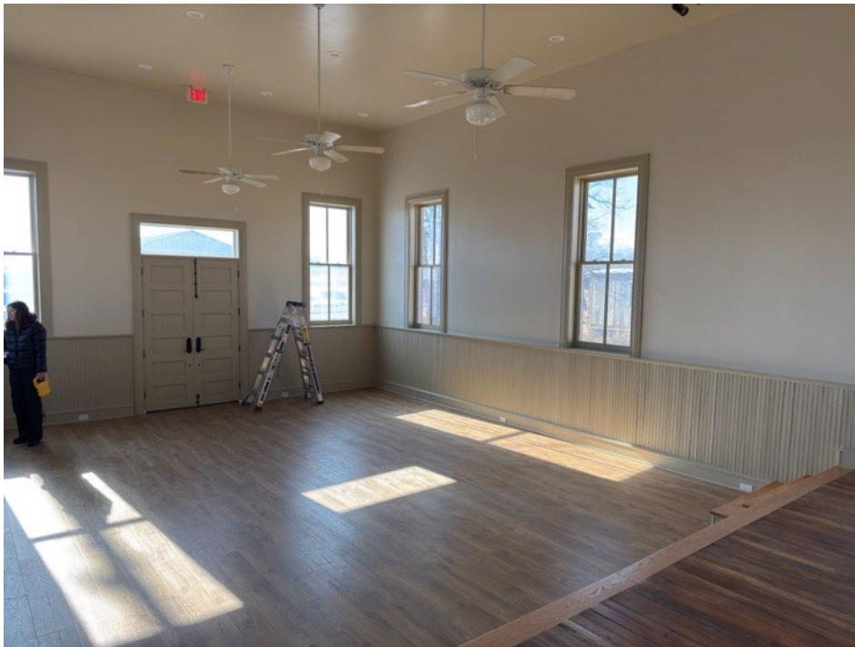
Photograph 14 of 19. Interior, showing wainscoting, windows, plaster, and replicated main entryway. Camera facing southwest.
