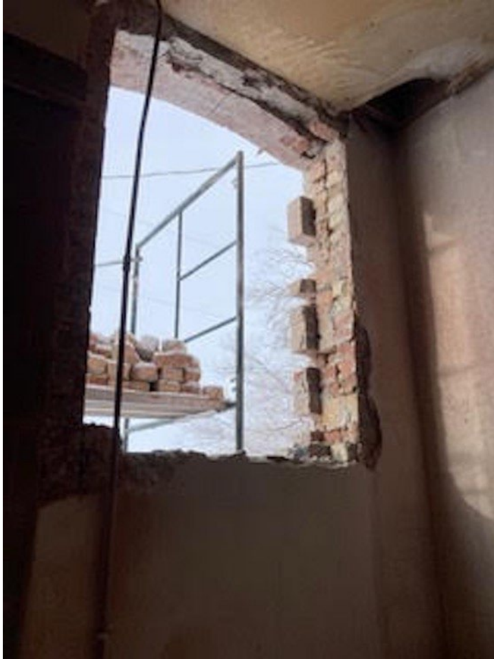
Figure 9 of 14. Interior photo of the south façade window restoration, ca. 2022. Camera facing south. Source: Clover Church Restoration Committee.
