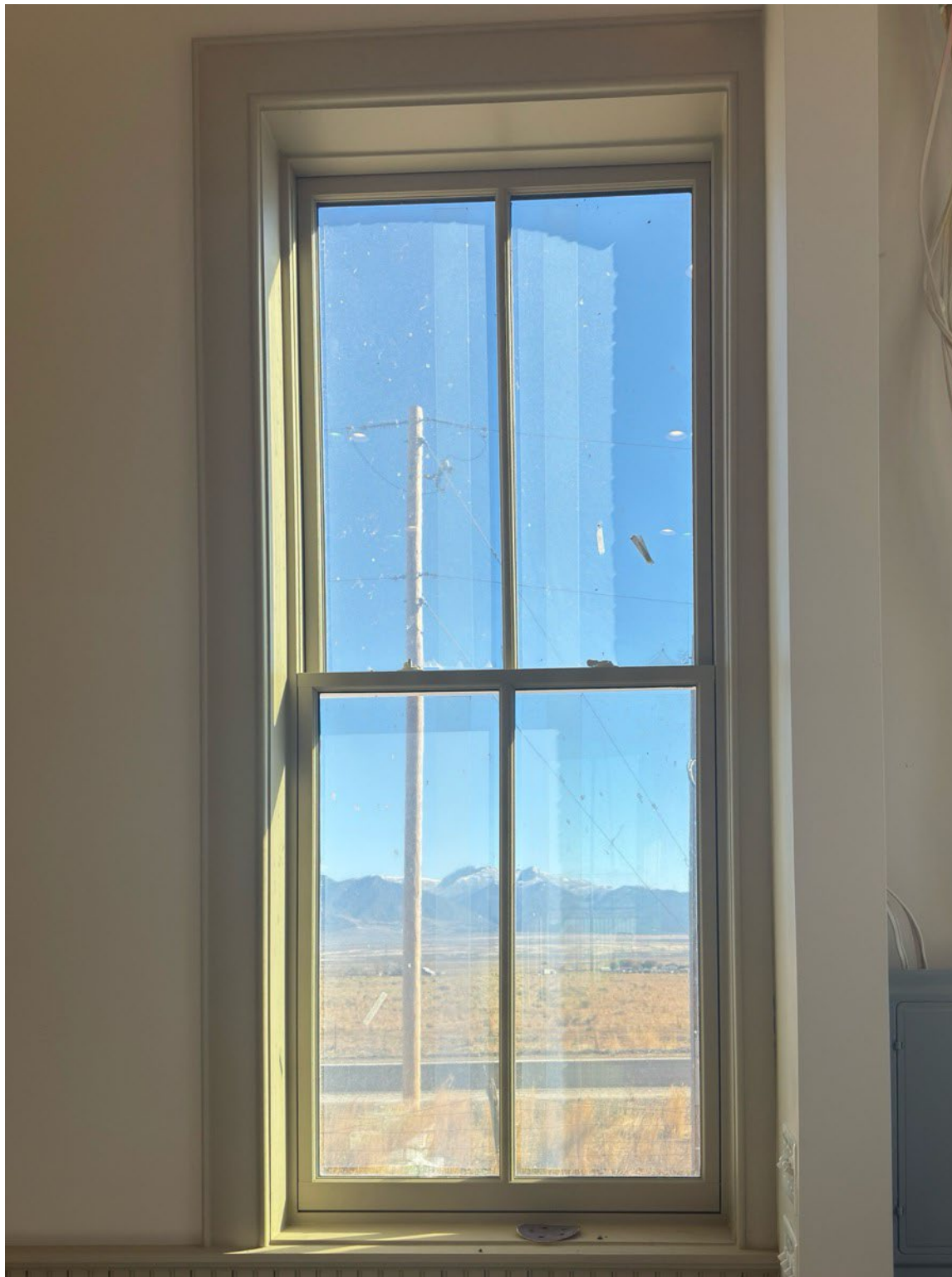
Photograph 16 of 19. Interior, detail of restored windows and power box can be seen to the right. Camera facing east.
