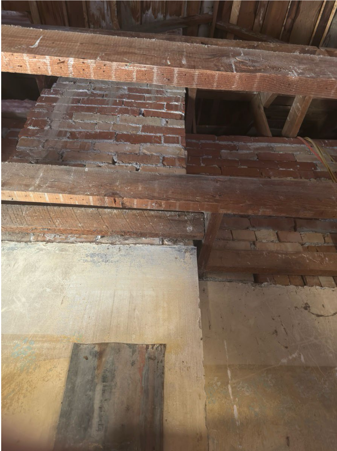
Photograph 19 of 19. Interior, vestry addition, detail of exposed rafters and original masonry. Camera facing up.
