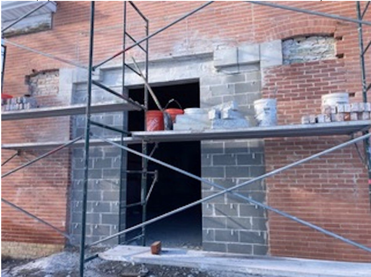
Figure 8 of 14. Restoration of the main (south) façade entryway, ca. 2022. Camera facing north. Source: Clover Church Restoration Committee.
