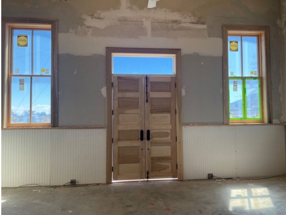
Figure 11 of 14. Interior renovations of the south façade, showing window and entryway replacements, ca. 2022. Camera facing south. Source: Clover Church Restoration Committee.
