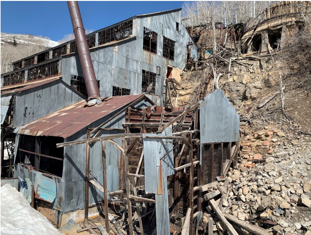
Photo No. 23 Detail of east elevation showing boiler room, chimney, coal bin and water tank. Camera facing north-west.
