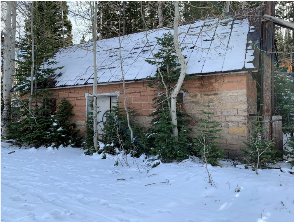
Photo No. 24 North (primary) elevation of the Transformer House. Camera facing south
