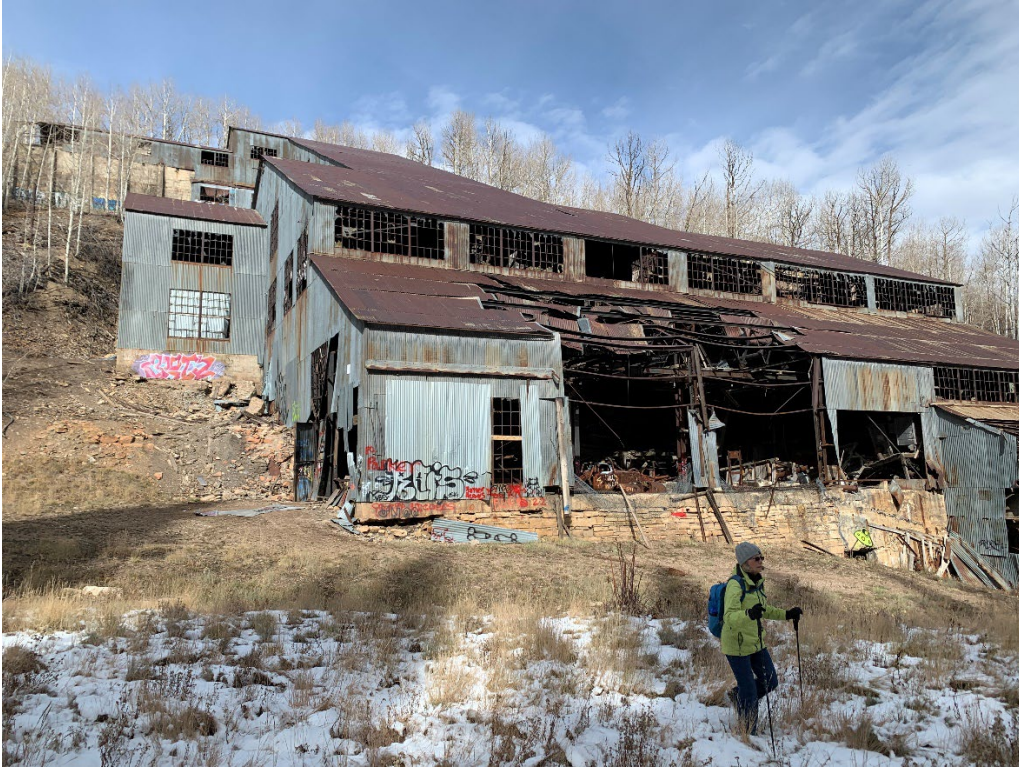
Photo No. 20 South and west elevations of Silver King Mill. Camera facing north-east.
