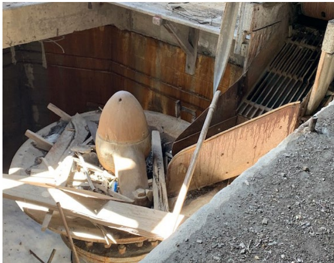
Figure 14. Allis-Chalmers gyratory crusher (full of wood and debris) and grizzly on the right. A grizzly is simply a screen with metal bars placed so smaller ore pieces could fall through and bypass the crusher.
