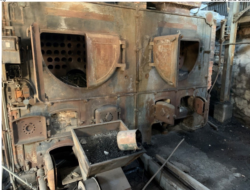
Figure 2. The two boilers located inside the Shaft House were abated for asbestos in 2023. Source: Sandra Morrison 2024.
