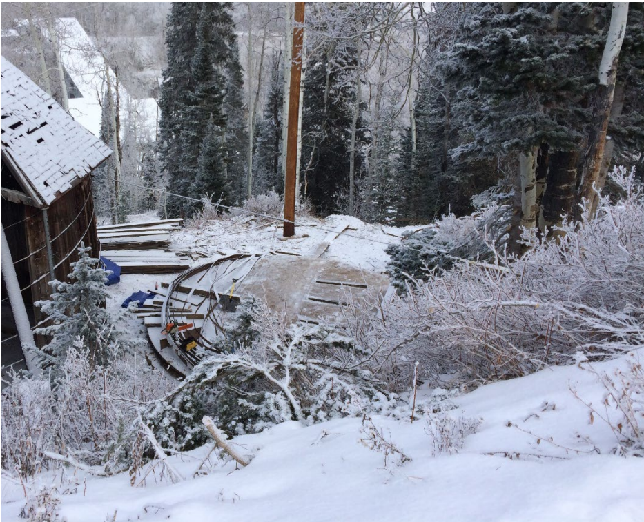
Photo No. 47 Remains of collapsed Water Tank C. Camera facing north.
