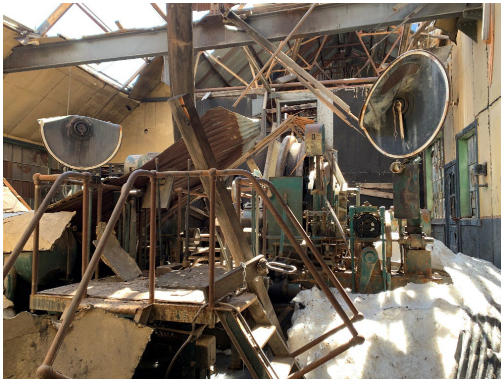
Figure 1. The 1937 Norberg electric hoisting equipment, including the reels and flat rope remain inside the Shaft House. The two (damaged) round gauges indicate on which level the cage is located.
