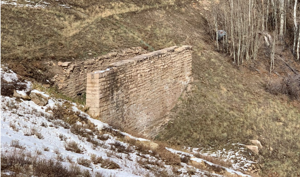
Photo No. 42 East elevation of Sampler Building Foundation Walls. Camera facing north.
