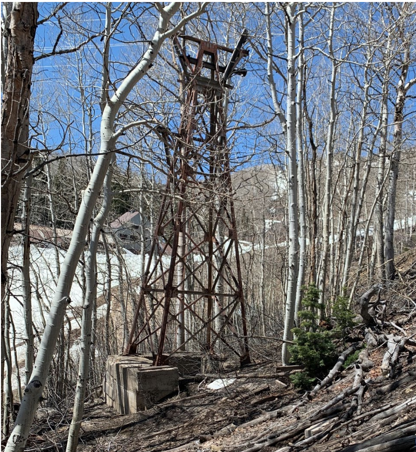
Photo No. 43 North elevation of Aerial Tramway Tower 39 with Shaft House in background. Camera facing south.
