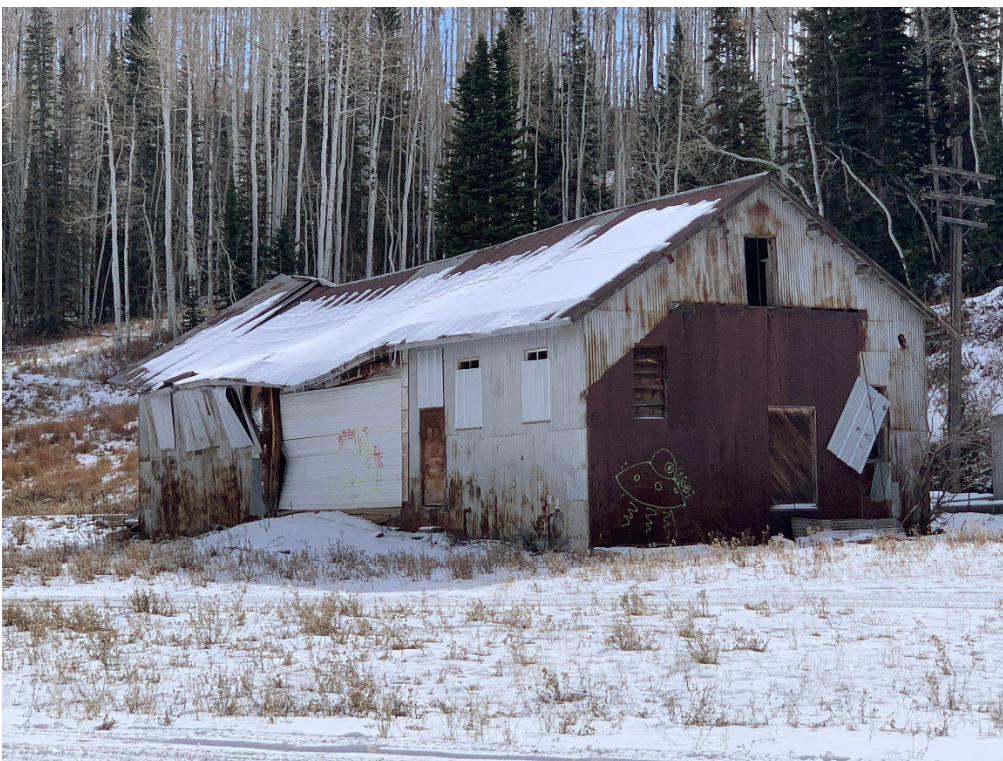
Photo No. 15 West and north elevations of the Warehouse. Camera facing south-east.
