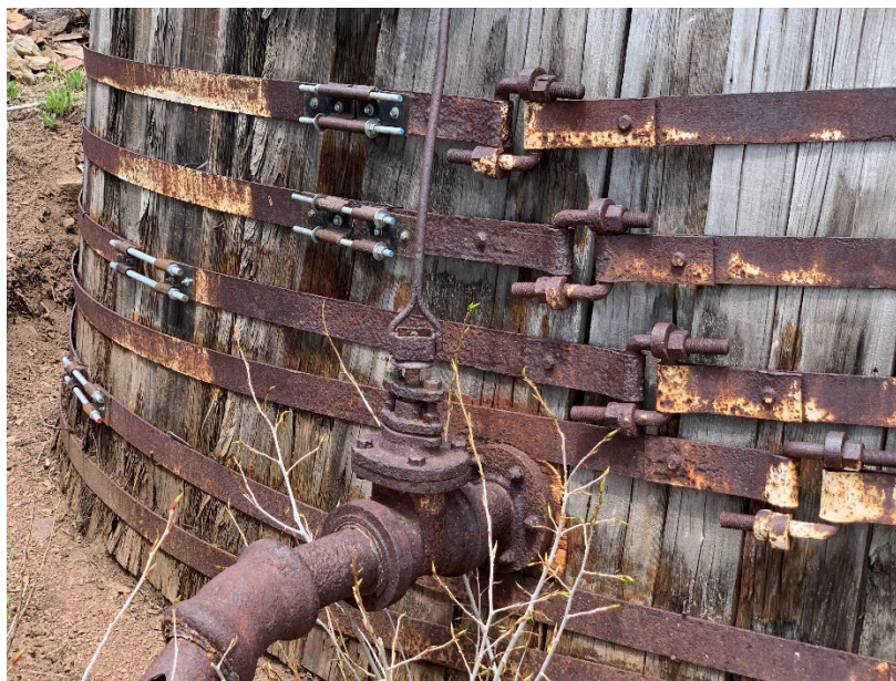
Figure 6. Metal bands with new closure hardware and drainpipe/valve on Water Tank A. Source: Sandra Morrison. 2024
