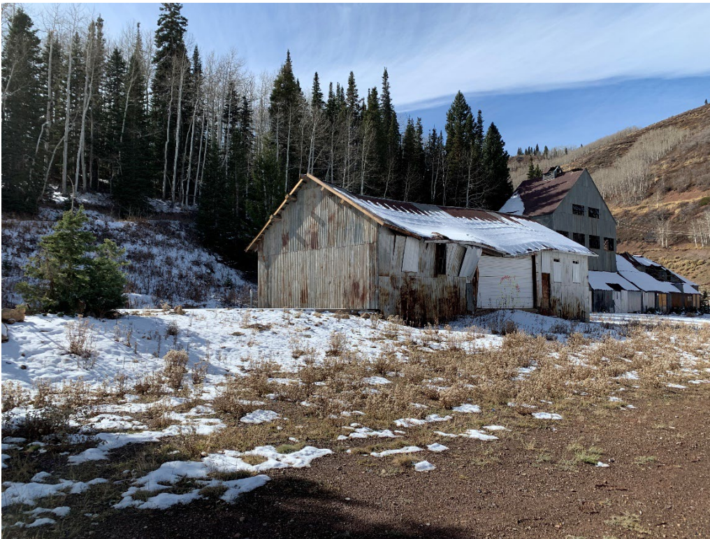
Photo No. 17 East and north elevations of the Warehouse with Shaft house in rear. Camera facing south-west
