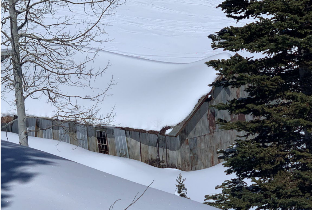
Photo No. 16 South and East elevations of the Warehouse. Camera facing north-west
