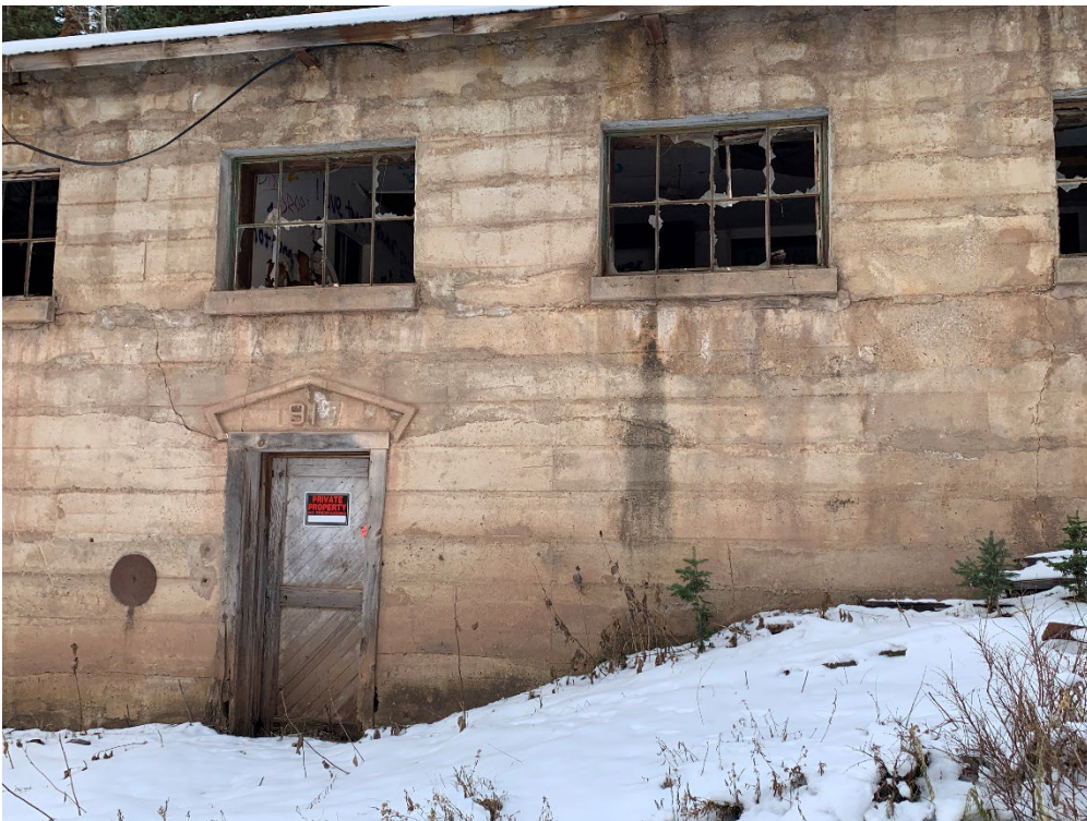
Photo No. 13 Detail of window and front door of the Change House. Camera facing south
