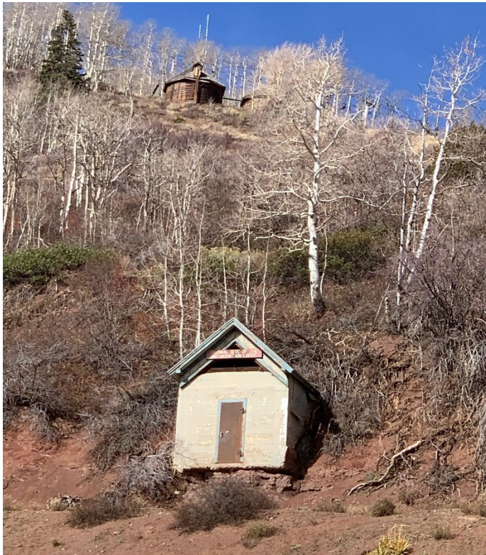
Photo No. 31 East elevation of Boarding House Vault with Water Tanks A & B uphill. Camera facing west.
