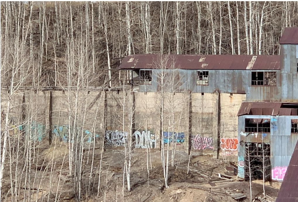
Photo No. 21 South elevation of Silver King Mill. Detail showing covered tramway with concrete ore loading bins below. Camera facing north.
