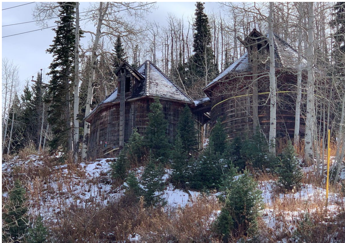
Photo No. 32 North elevation of water Tanks C, D & E. Camera facing south
