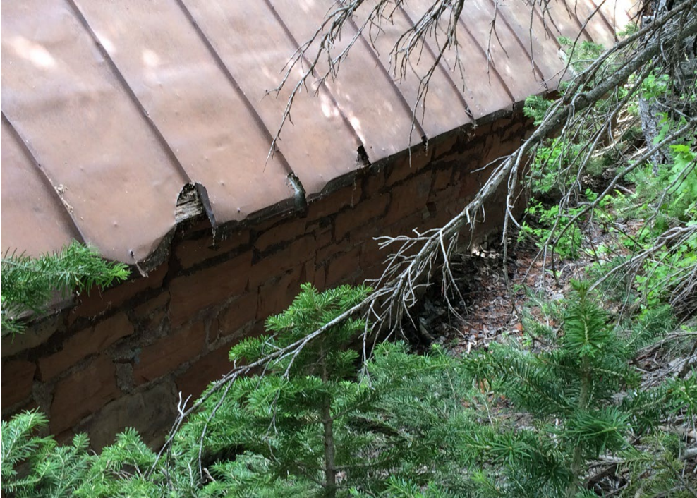
Photo No. 26 South elevation (constructed into the hillside of the Transformer House. Camera facing north
