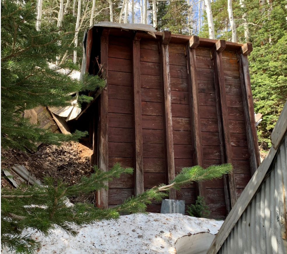
Photo No. 28 Coal bunker with corner of Shaft House visible on right. Camera facing south.
