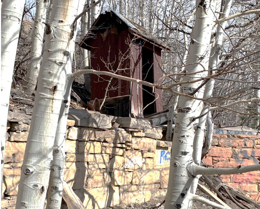
Photo No. 40 South elevation of Mill Fire Hose Shack 1 and stone wall. Camera facing north
