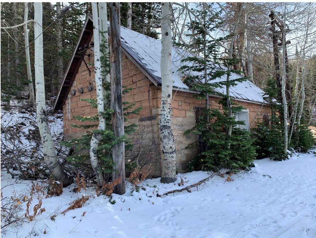
Photo No. 25 East and north elevations of the Transformer House. Camera facing southwest.
