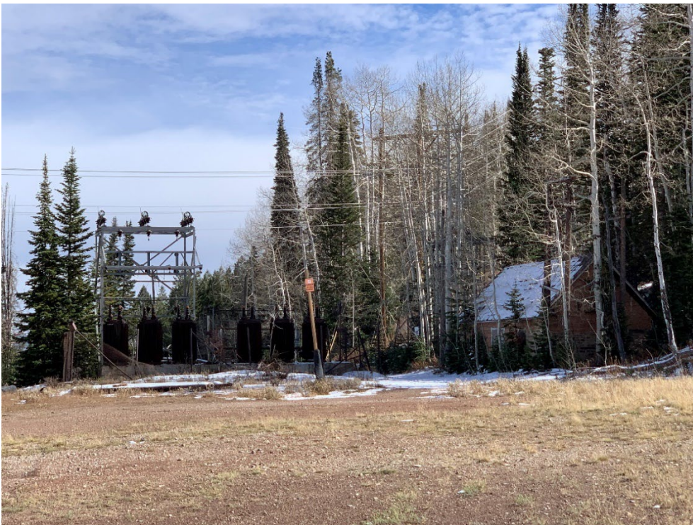
Photo No. 27 Overview of waste rock dump, transformer house and substation located east of the shaft house. Camera facing east.
