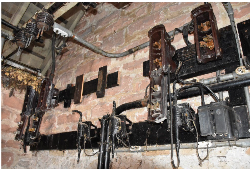
Figure 5. Switches and equipment located inside the Transformer House. Source: Sandra Morrison. 2024.
