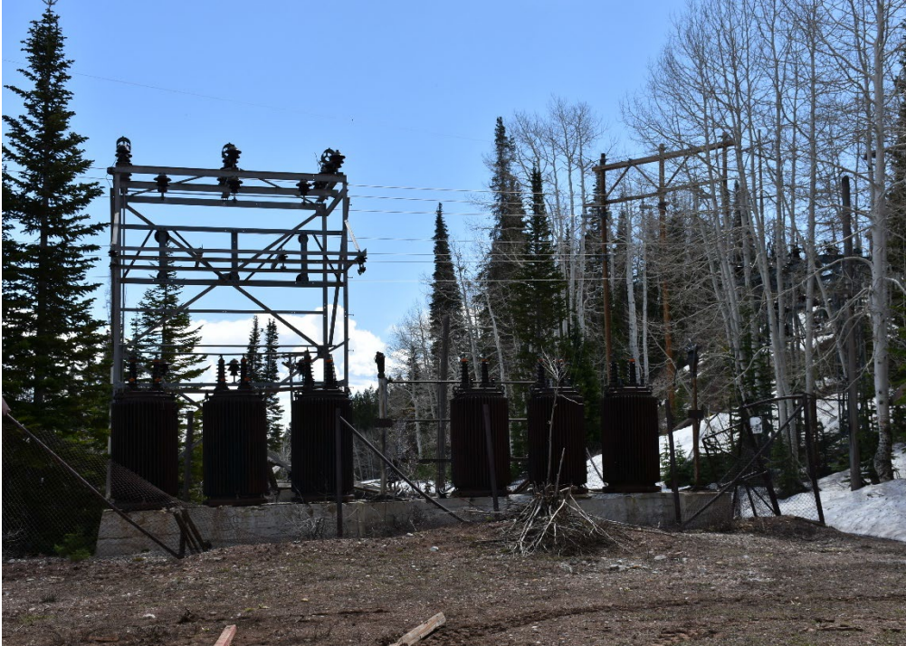
Photo No. 44 East elevation of Surface Transformer Substation. Camera facing east.
