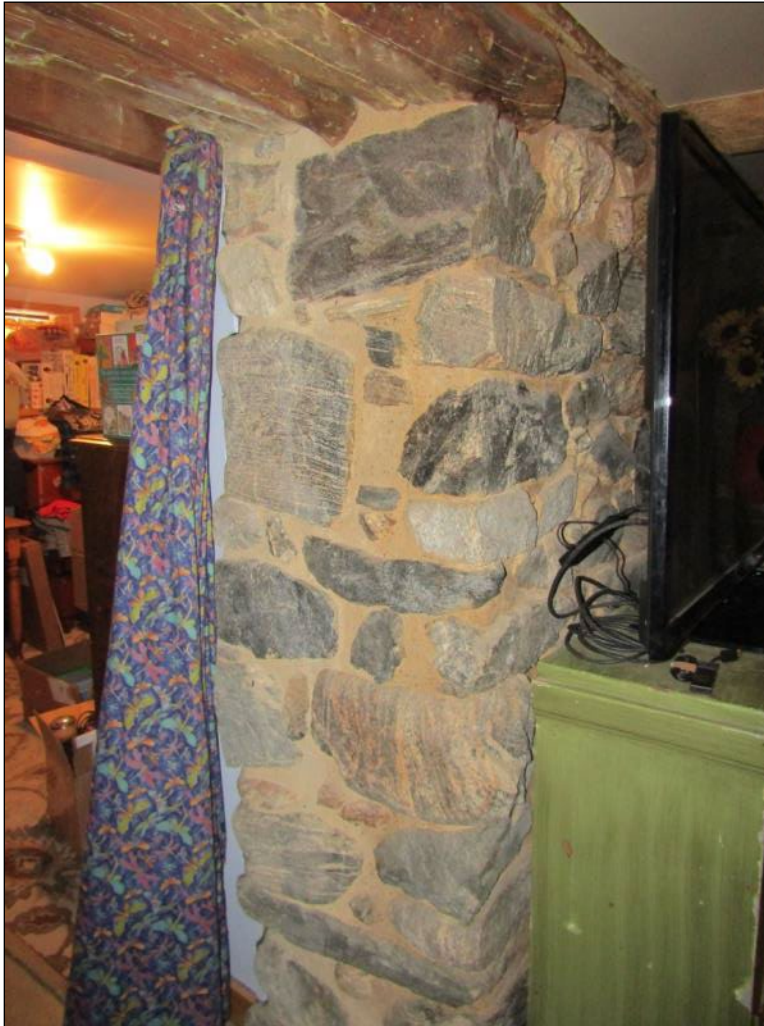
Photograph 14. Interior – basement showing thickness of interior walls and raw timber floor joists; camera facing north-northwest
