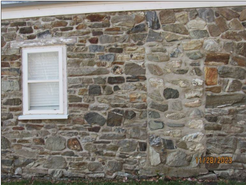
Photograph 8. Infilled original doorway and window opening in east elevation; camera facing west
