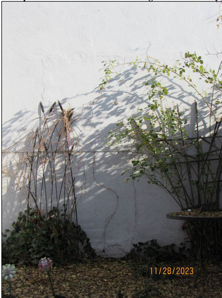
Photograph 9. Crack in plaster of west elevation showing former doorway; camera facing east
