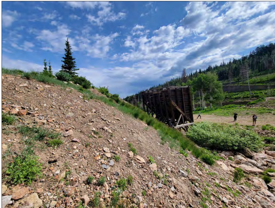
Photo No. 8 Overview of ore bin and waste rock dump. Camera facing northwest.
