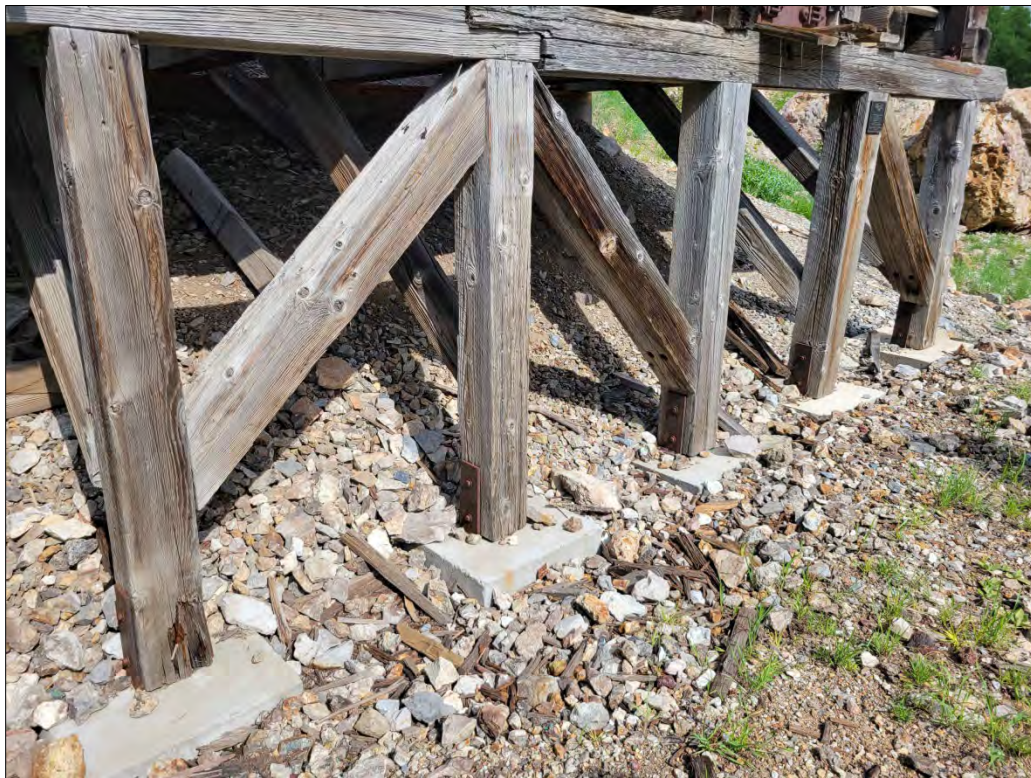
Photo No. 5 Detail of support posts and concrete piers. Camera facing northwest.
