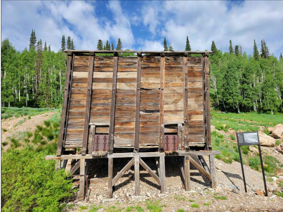
Photo No. 2 East (primary) elevation of the Little Bell ore bin. Camera facing west.
