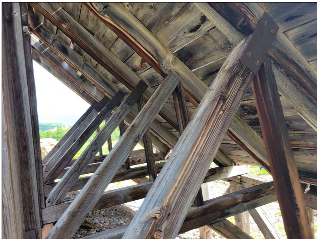
Photo No. 9 Detail of cross-brace timbers, sloped floor and mortise-and-tenon joints. Camera facing northwest.
