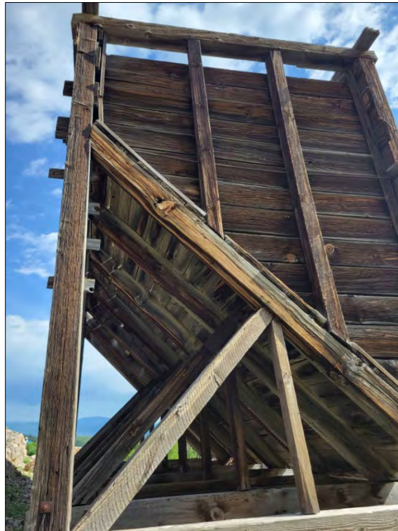
Photo No. 7 South elevation detail showing cross brace timbers. Camera facing north.
