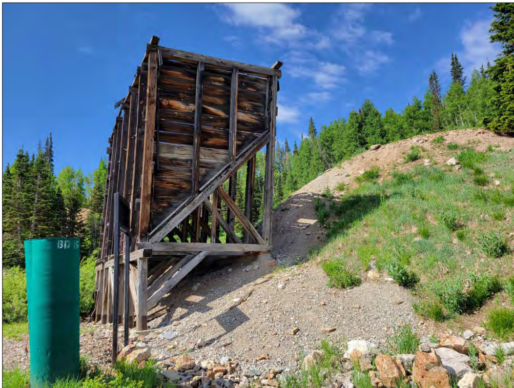
Photo No. 11 North elevation of ore bin and waste rock dump. Camera facing south.
