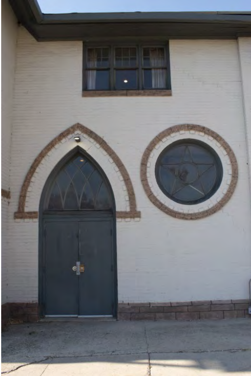
Photograph 5 of 35. Exterior, Phase I east elevation detail showing door and window detail. Camera facing west.
