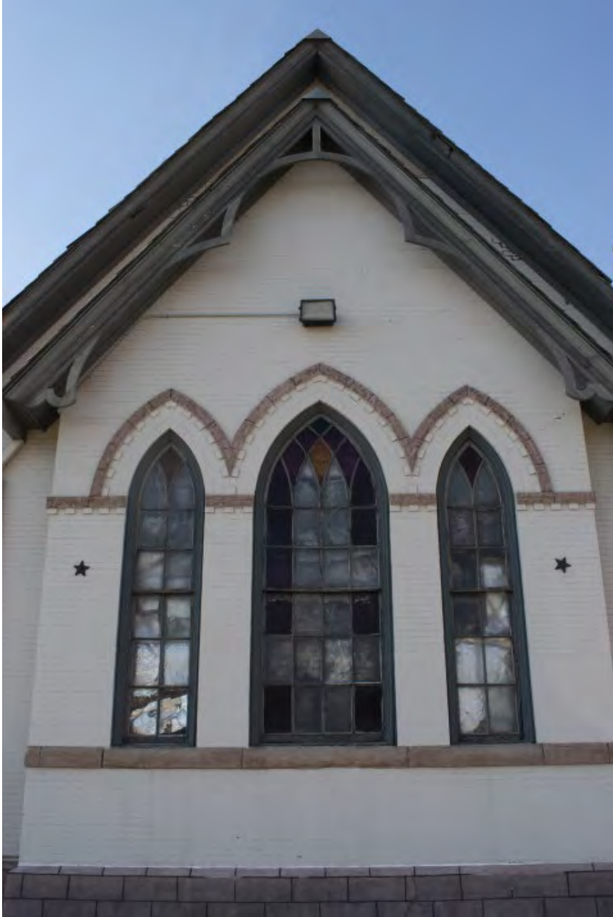
Photograph 6 of 35. Exterior, Phase I east elevation detail showing window and gable detail. Camera facing west.
