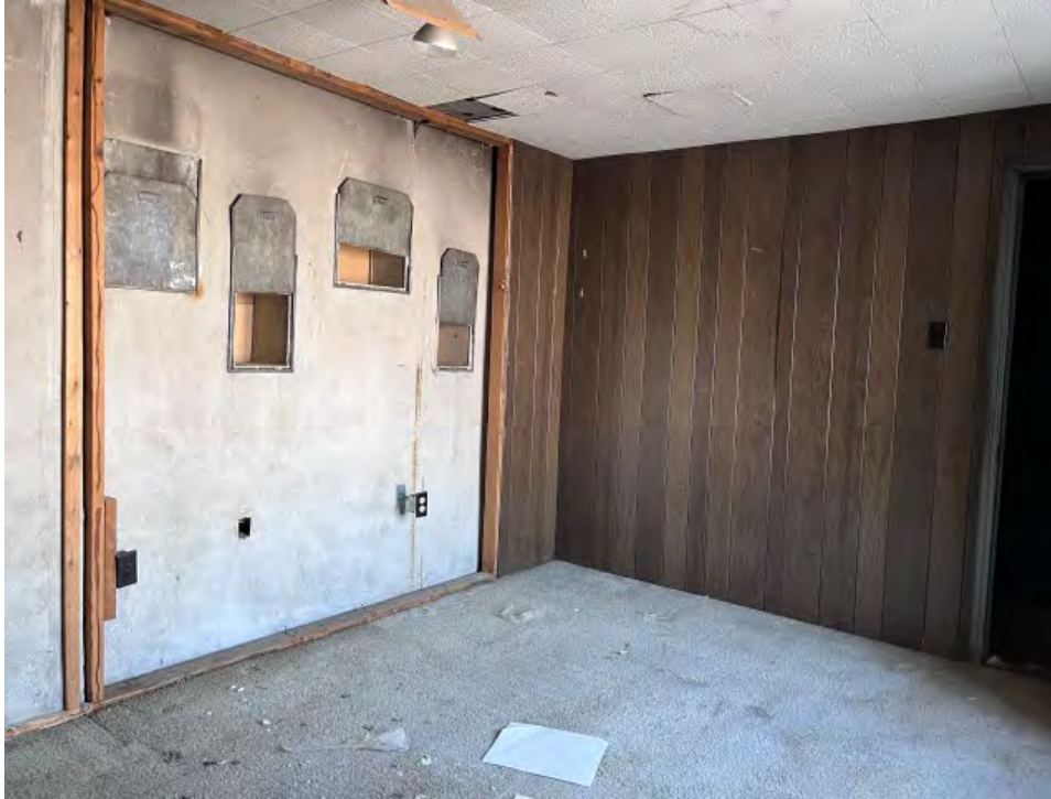
Photograph 29 of 35. Interior, Phase II second floor projection room showing wall openings. Camera facing southwest.
